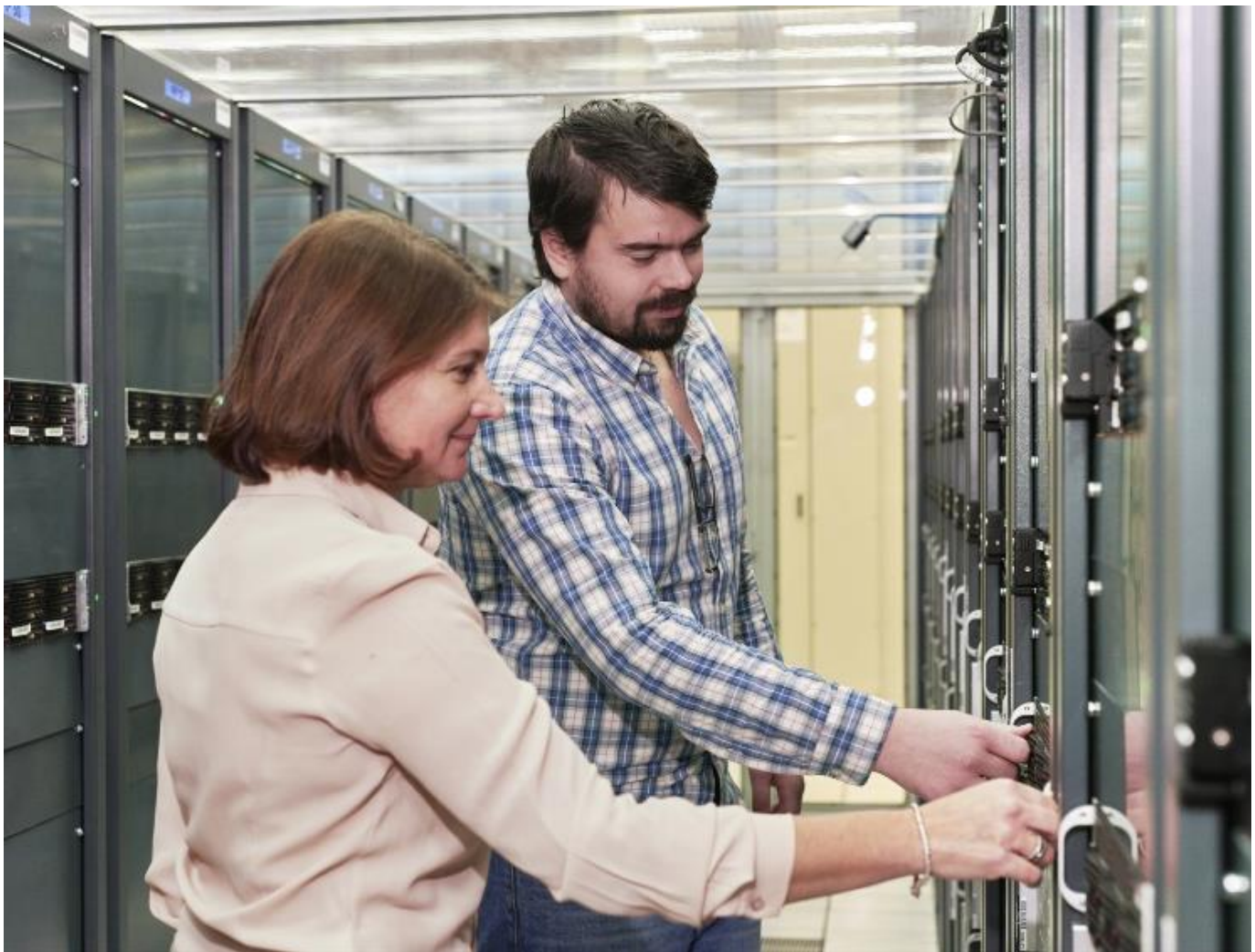
Maria Girone and Viktor Khristenko, CERN members of the project team, pictured in the CERN data centre.
